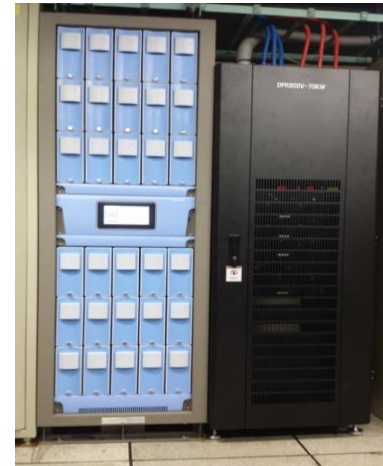
[ East Jinju base station ]
