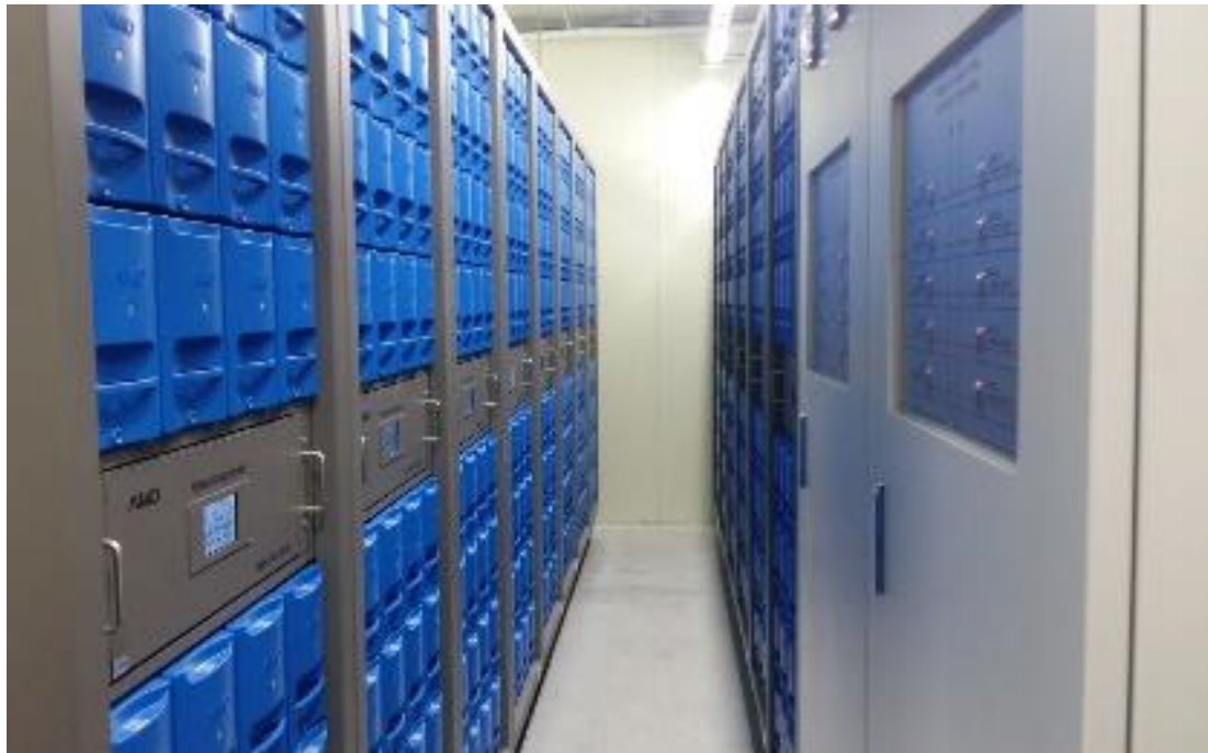
Battery + PCS (1MWh, 14 Rack)
