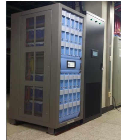
[ Chungcheong base station ]
