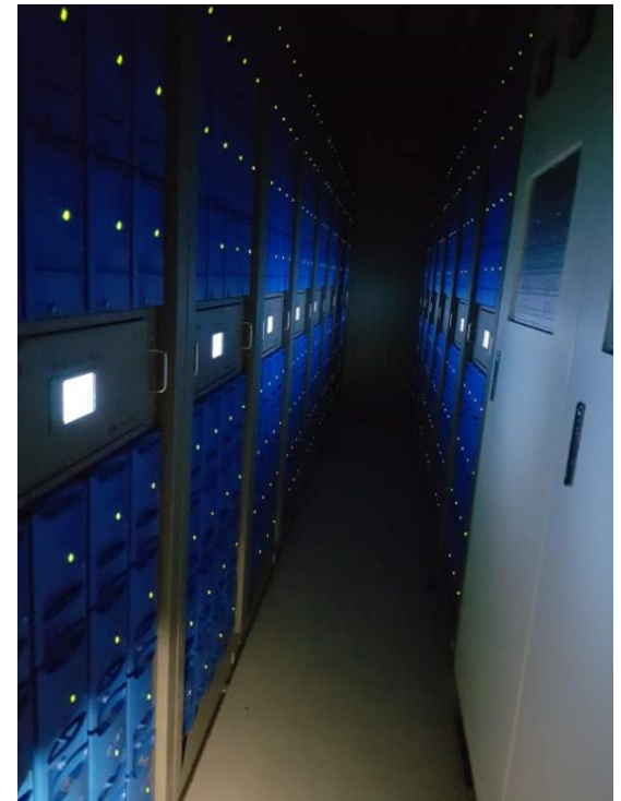
Battery + PCS (1.5MWh, 21 Rack)
